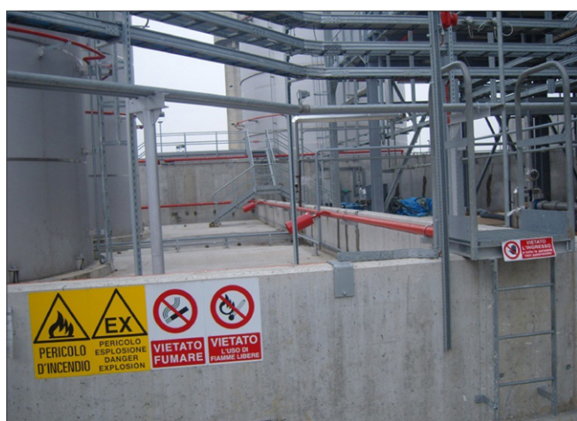
Fig. 3 - Fixed foam monitors
